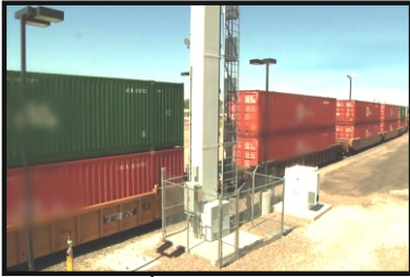
Radiation Monitoring System
